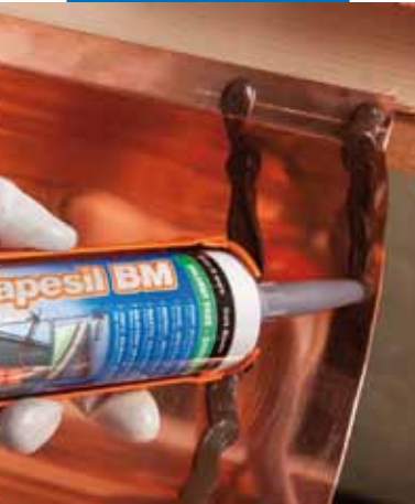
Extruding Mapesil BM on the lower sheet of metal before overlaying with another sheet
